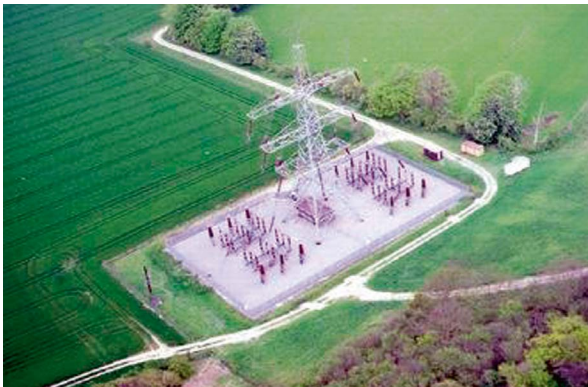
A typical sealing end compound for a directly buried cable
