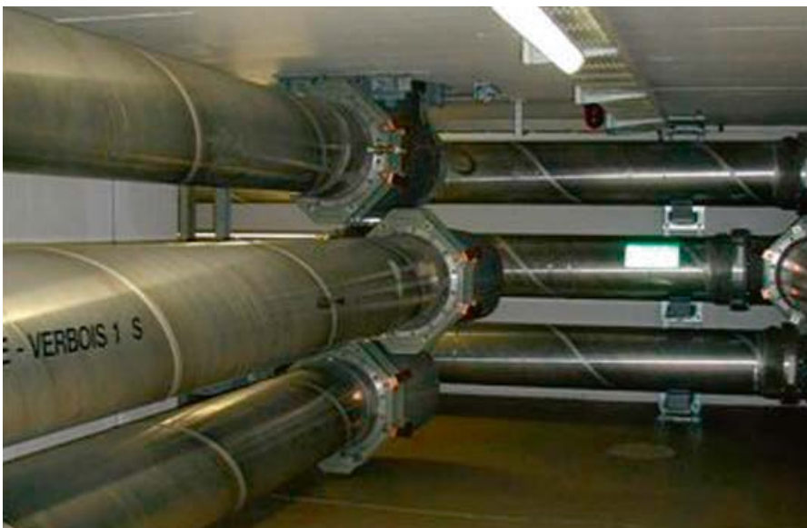
Gas insulated lines installed in tunnel
